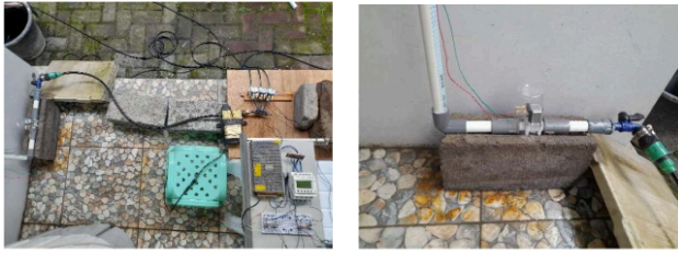
Figure 3.9 PLC Installation, Figure 3.10 PLC Installation, main valve
