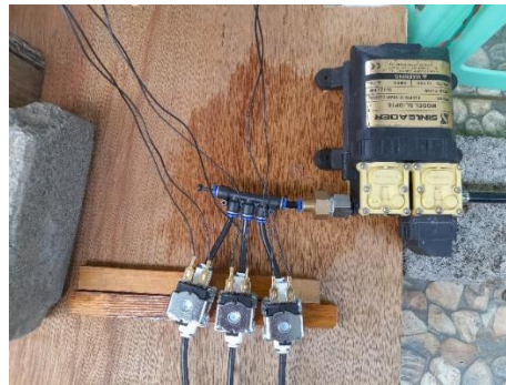
Figure 3.11 Garden solenoid installation
